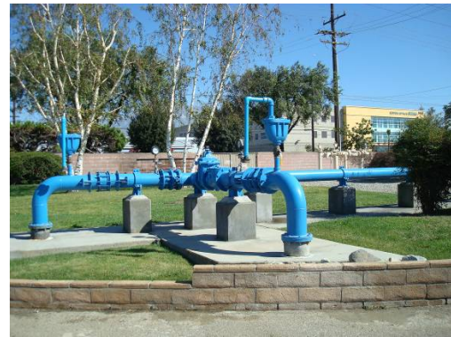
The New ASR Well suction and discharge pipe design would connect above grade.
