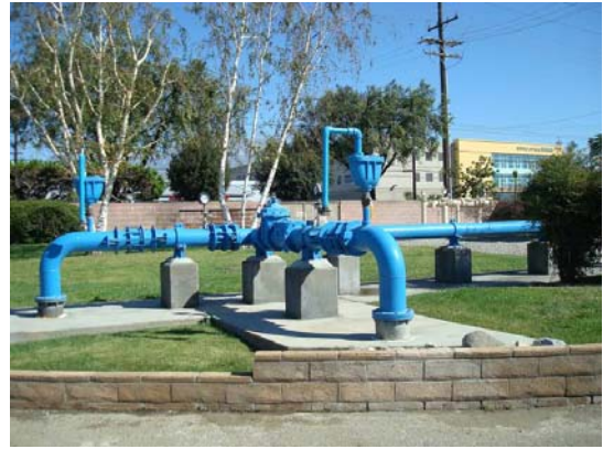
Existing Well No. 4 discharge piping will need to be modified to tie into the new plant.
