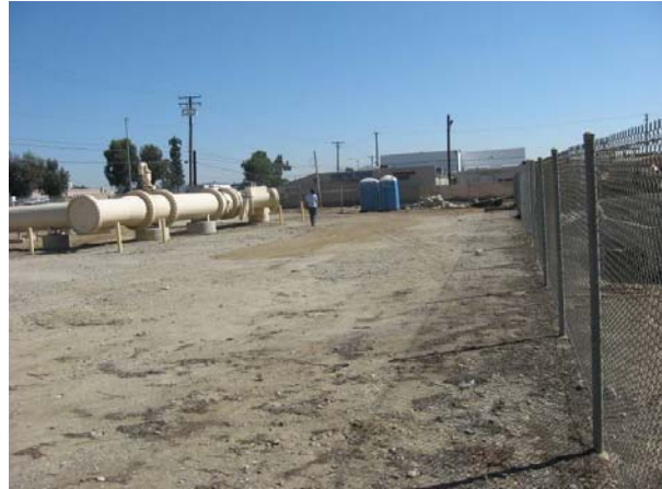
The New ASR Well site has space constraints due to existing above-grade piping for the new IX and well facilities.
