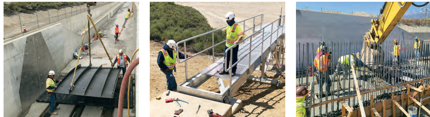
The Lower Day Improvement Project under construction. The completed project will increase stormwater diversion and Basin storage.
