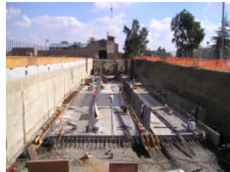
RP-1 Chlorine Contact Basin
