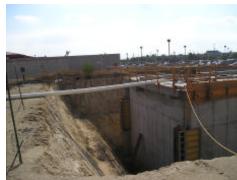
RP-1 New Pump Station
