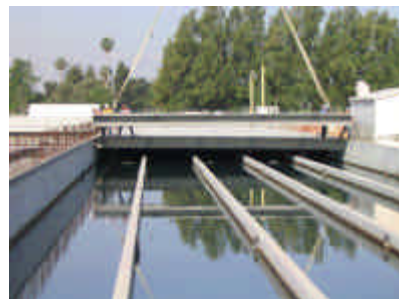
RP-1 New Chlorine Contact Basin
