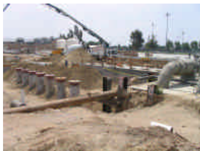
RP-1 New Pump Station
