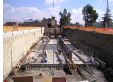
RP-1 Chlorine Contact Basin
