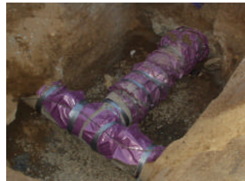
Pine Avenue Intertie Phase I
