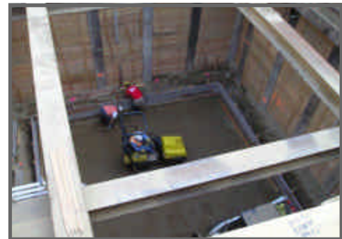
Jurupa Pump Station
