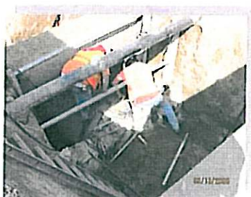
RP-4, 1158 Pipeline, Segment A
