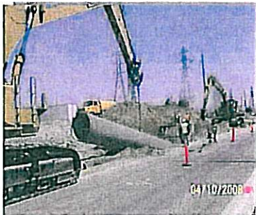
RP-4, 1158 Pipeline, Segment A
