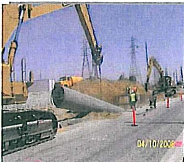
RP-4, 1158 Pipeline, Segment A
