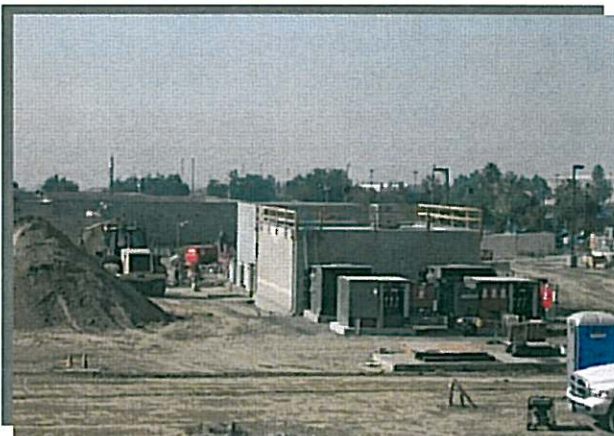
RP-4 1158 Reservoirs, Pump Stations, and Pipeline
