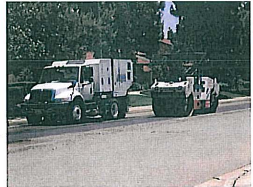
San Antonio Channel Pipeline, Segment B
