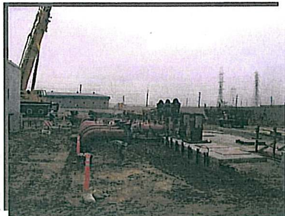
RP-4 1158 Reservoirs, Pump Stations, and Pipeline
