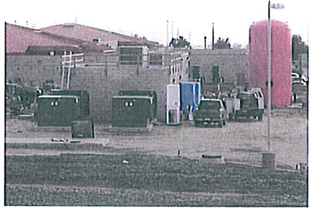
1299 Electric Bldg, Surge Tank and Pump station
