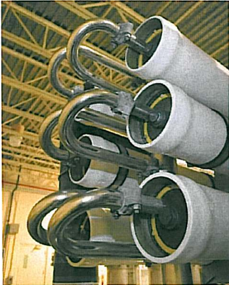
Reverse osmosis equipment used in desalting facilities.
