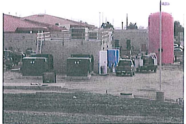
1299 Electric Bldg, Surge Tank and Pump station
