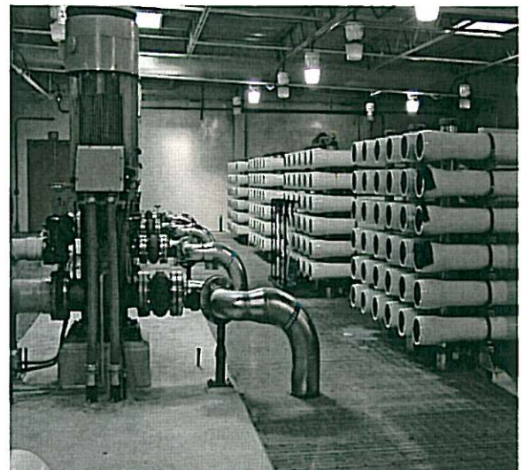
Chino Desalter I Feed Pumps and RO Membranes
