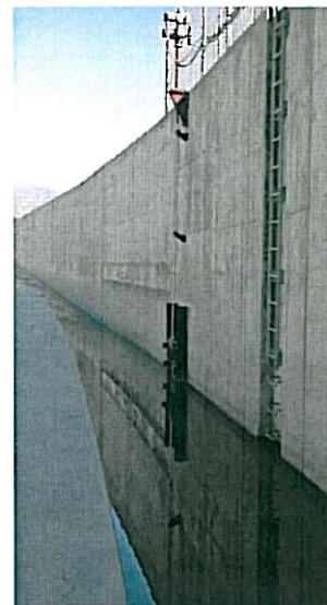
New inlet gate in San Sevaine Channel to Jurupa Basin
