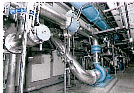
Pumps and pipes at the Orange County Water District move treated effluent through the plant as it becomes ultra pure water, in Fountain Valley, Ca.
