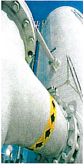
Desalter Product Water Tank
