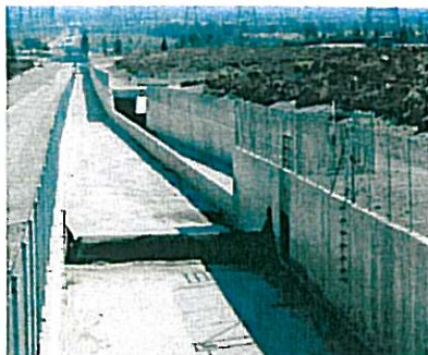
Rubber dam inflated near Lower Day Basin
