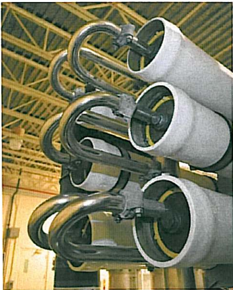
Reverse osmosis equipment used in desalting facilities.
