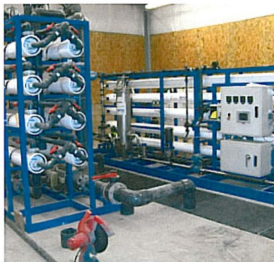
Photo: Tom Stewart Highly purified RO is one step in the process to turn wastewater into a purified product.
