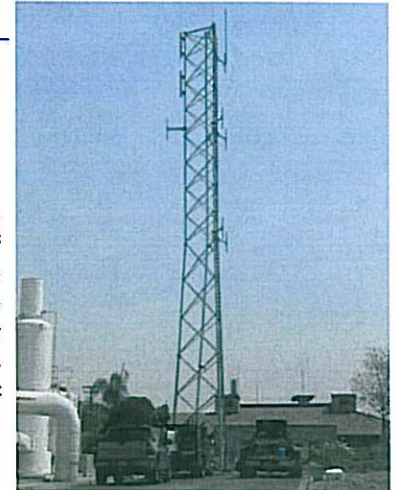
New Radio Antenna for the SCADA system
