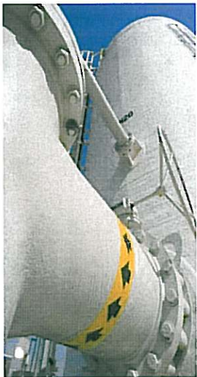
Desalter Product Water Tank
