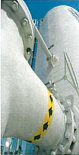
Desalter Product Water Tank
