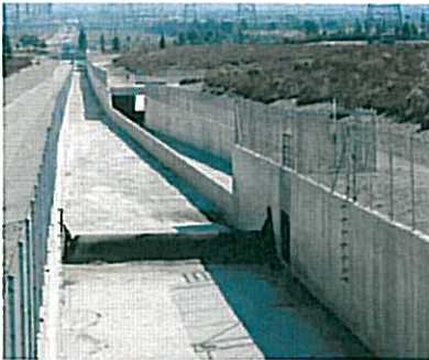
Rubber dam inflated near Lower Day Basin
