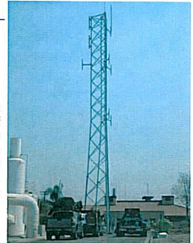
New Radio Antenna for the SCADA system
