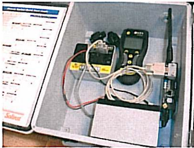
New Telemetry system being tested
