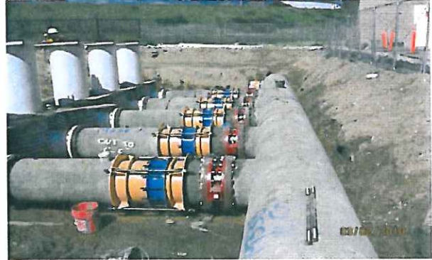
1630 E. Pump Station
