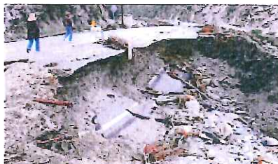
A portion of Lytle Creek Road is washed out. (Will Lester Staff Photographer)
