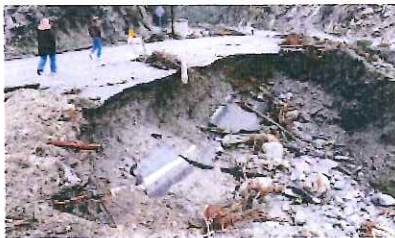
A portion of Lytle Creek Road is washed out. (Will Lester Staff Photographer)
