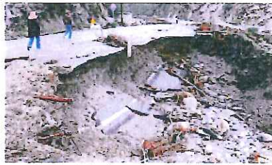
A portion of Lytle Creek Road is washed out. (Will Lester Staff Photographer)
