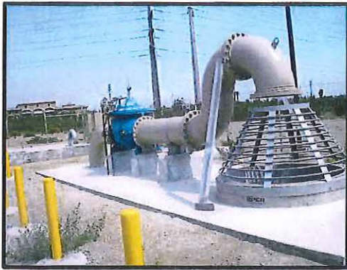
CB-20 Turnout Facility
