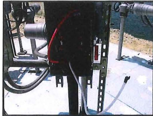
Damages to new electrical enclosure
