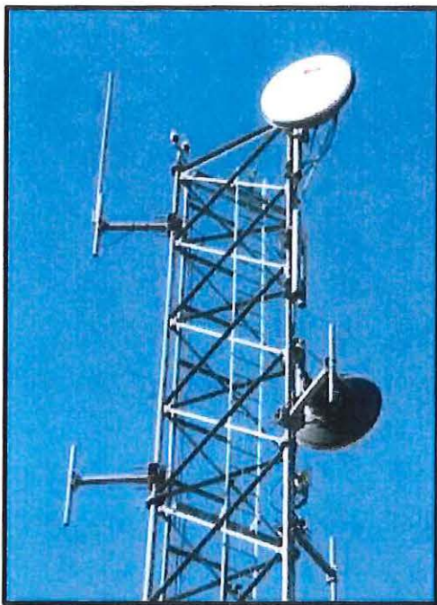
Basin Communication Tower
