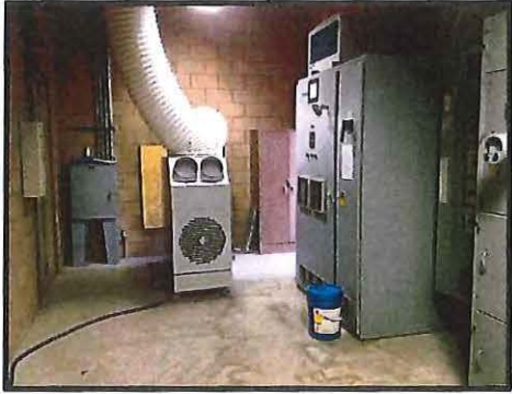
MCC Control Panel
