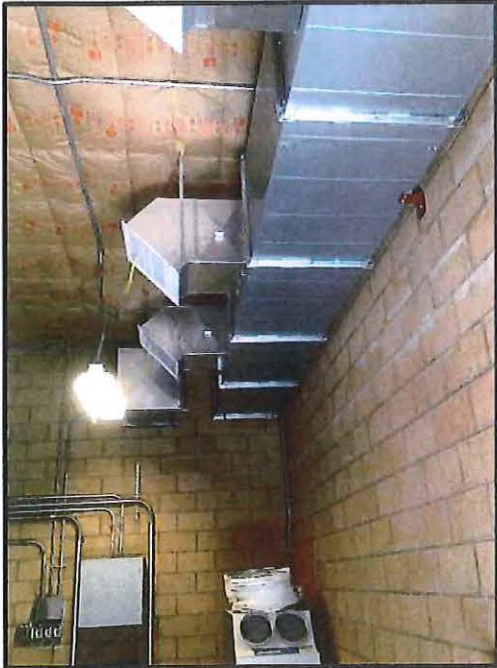
Installed ceiling insulation and AC air ducting
