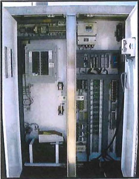
San Sevaine turnout control panel
