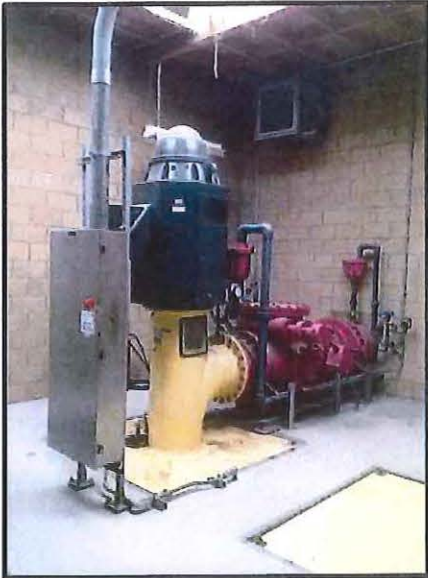
Existing pumping system
