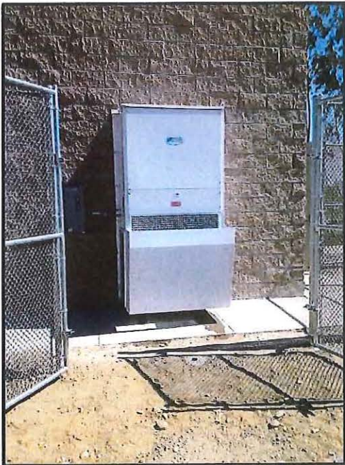
Installed AC unit
