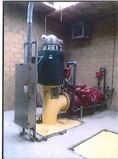
Existing pumping system
