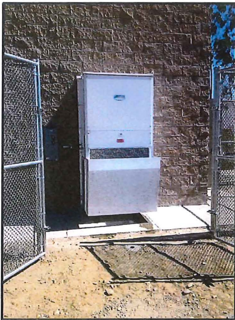
Installed AC unit
