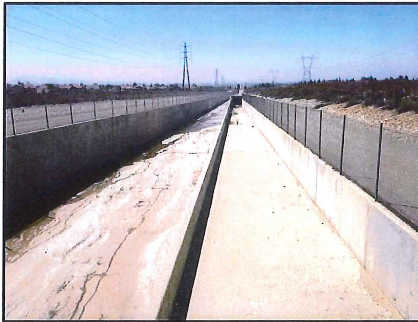
Field photo showing the location of the proposed improvement to the existing channel to increase storm water capture
