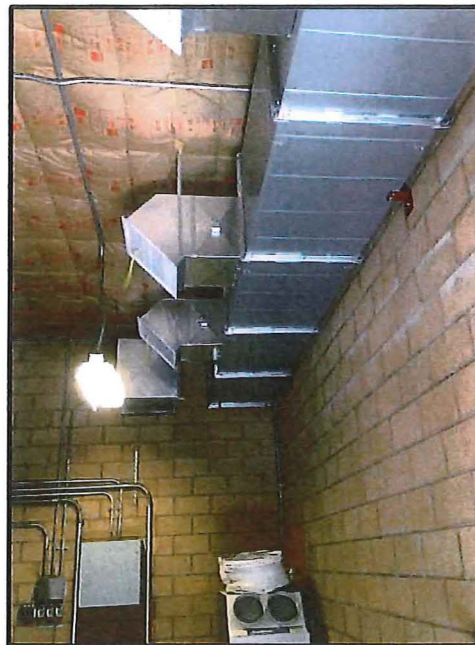
Installed ceiling insulation and AC air ducting
