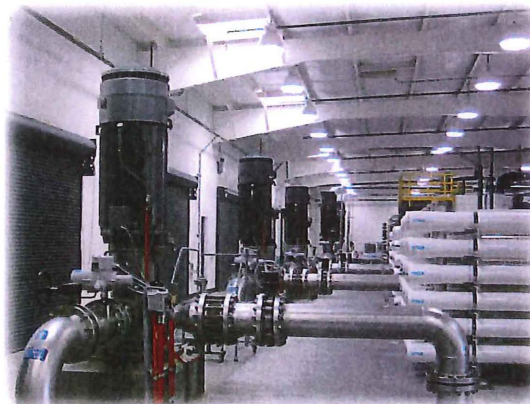
Chino Basin Desalter Authority Plant #2
