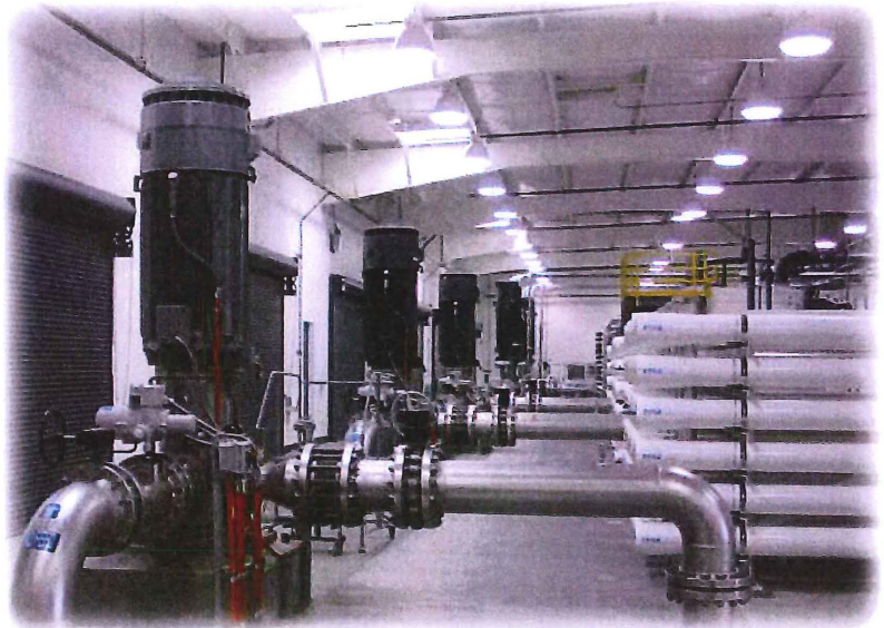
Chino II Desalter Facility
