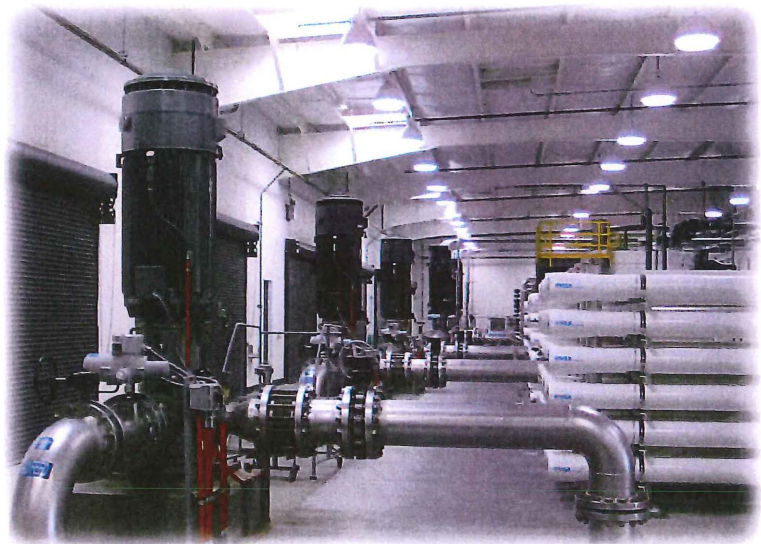
Chino II Desalter Facility
