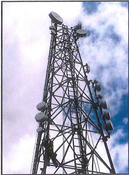
6B Tower – New Receiving Dishes
