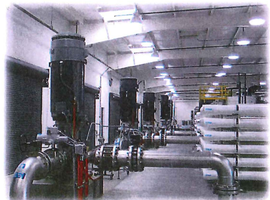
Chino Basin Desalter Authority Plant #2
