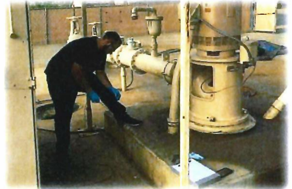
Maintaining Transducer Equipment in One of the Well Sites
