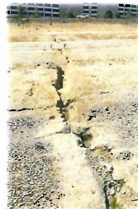
Fissuring at Ely Basin 3
