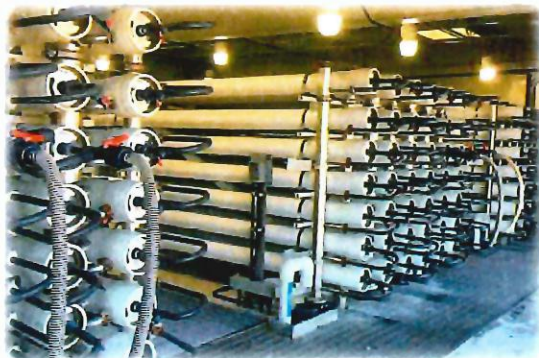
Chino Desalter I Facility
