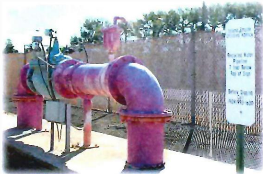
Recycled water line at the Ely Basins.
