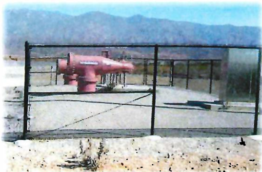
Recycled Water Line at the San Sevaine Basins
