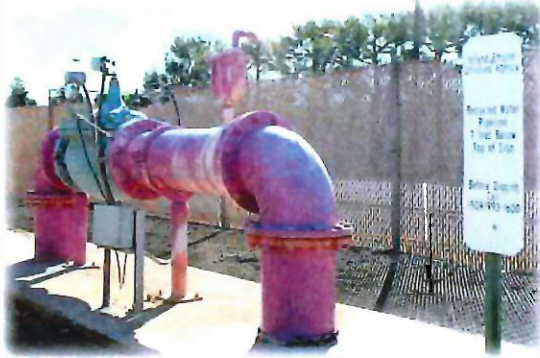
Recycled water line at the Ely Basins.
