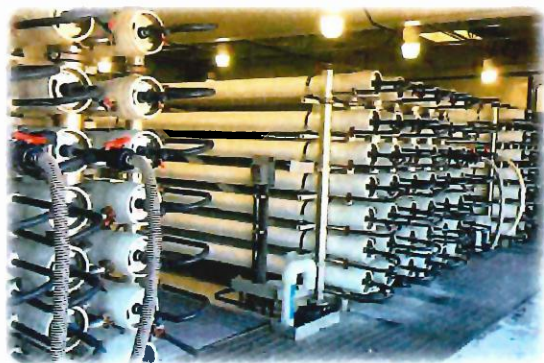
Chino Desalter I Facility
