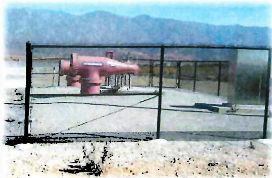
Recycled Water Line at the San Sevaive Basins
