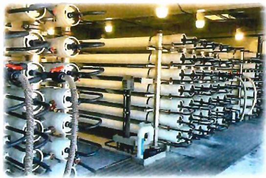
Chino Desalter I Facility
