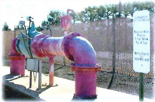
Recycled water line at the Ely Basins.
