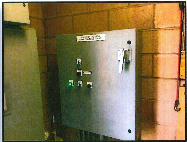
Rubber Dam control panel
