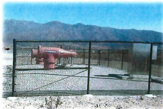
Recycled Water Line at the San Sevaime Basin #5.
