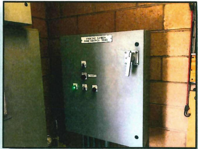
Rubber Dam control panel
