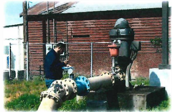
Reading a Meter on an Agricultural Well
