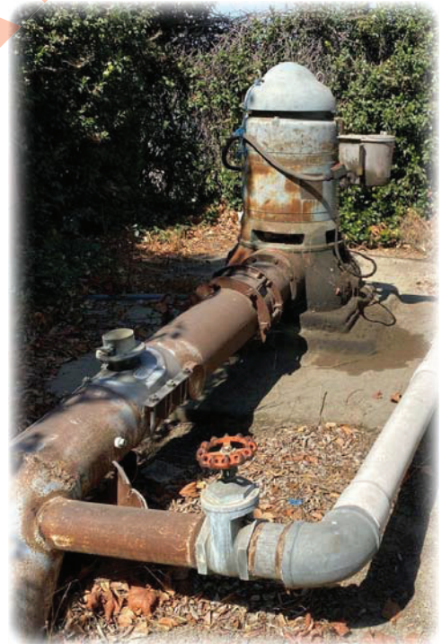
Metered Irrigation Well
