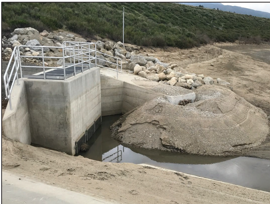
Discovered Alluvial Deposits near the New Stormwater Inlet Structure
