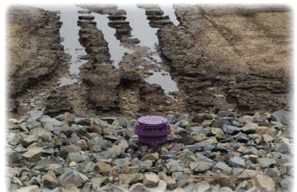
Recycled Water Outlet at San Sevaine Basin, Cell #2
