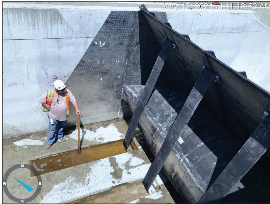
Lower Day's Main Channel – New Stormwater Diversion Gate
