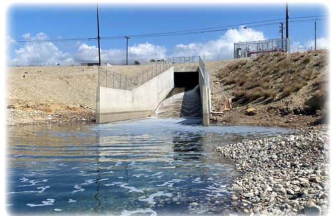
Recycled Water Being Discharged Into 8th Street Basin for Recharge
