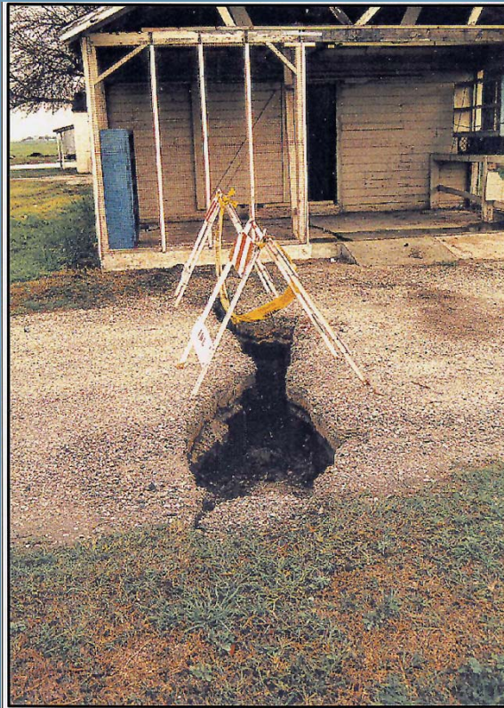
View of a fissure that developed beneath CIM facility in December 1992
