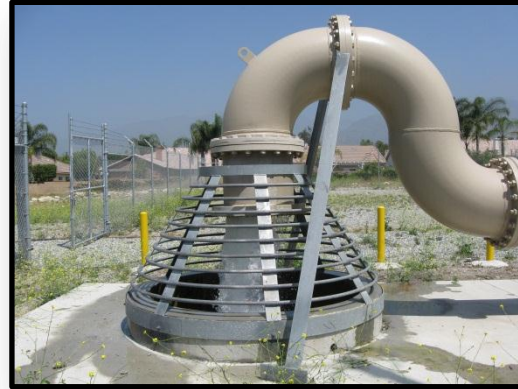
CB20 Outlet while in use
