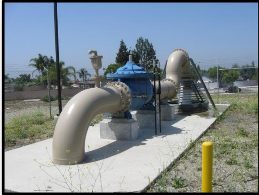
CB-20 Turnout Facility
