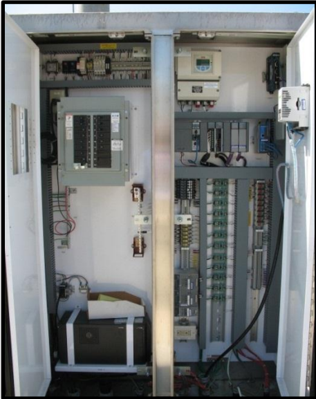
San Sevaine Turnout Control Panel
