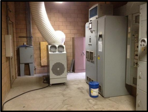
MCC Control Panel
