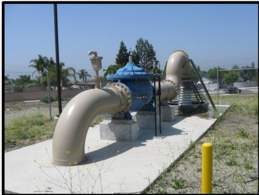
CB-20 Turnout Facility
