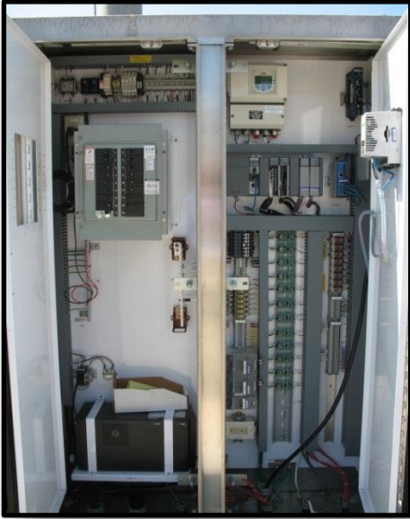
San Sevaine Turnout Control Panel
