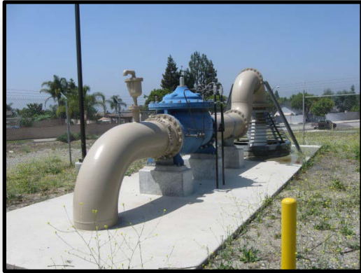
CB-20 Turnout Facility
