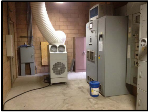
MCC Control Panel
