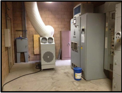
MCC Control Panel
